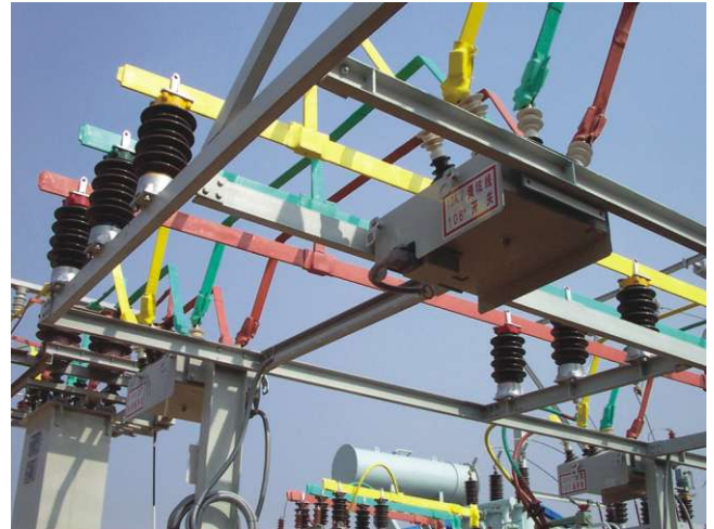
These 15kV reclosers are all networked back to the substation control room using MODBUS over a multi-dropped RS485 network.
