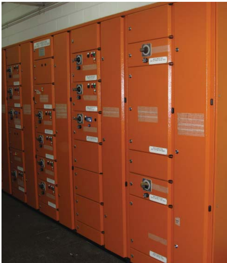
MCCs currently on site at Abbot Point
